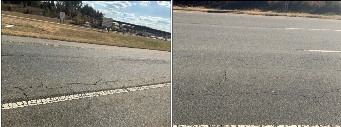
Figure 3: Paved Lanes Asphalt Inspection Results Sample
