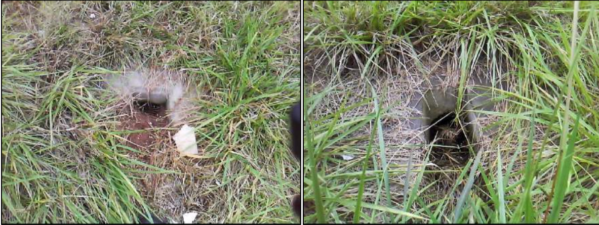
Figure 4: Miscellaneous Drainage Inspection Results Sample
